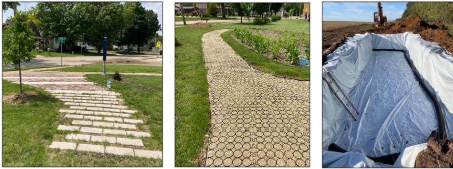
Charles City Sponsored Project: Edible arboretum entryway with limestone and brick pavers (left). Arboretum walkway of grass-gravel pavers (center). Denitrifying bioreactor installation (right).
